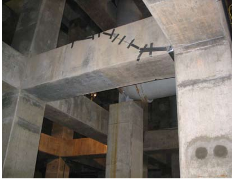
The pump station cracked like the spine of a book.
